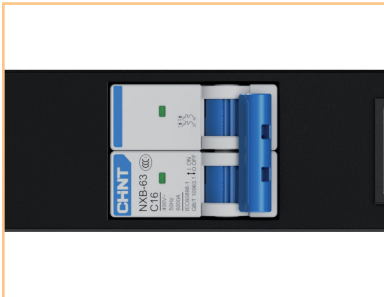
Overcurrent and short circuit protection by 16A circuit breaker
